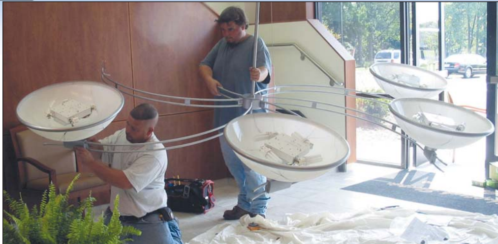
PRACTICING WHAT WE PREACH — Workmen install the chandelier in the lobby of the Denton headquarters. The fixture holds 24 compact fluorescent energy-saving bulbs.
